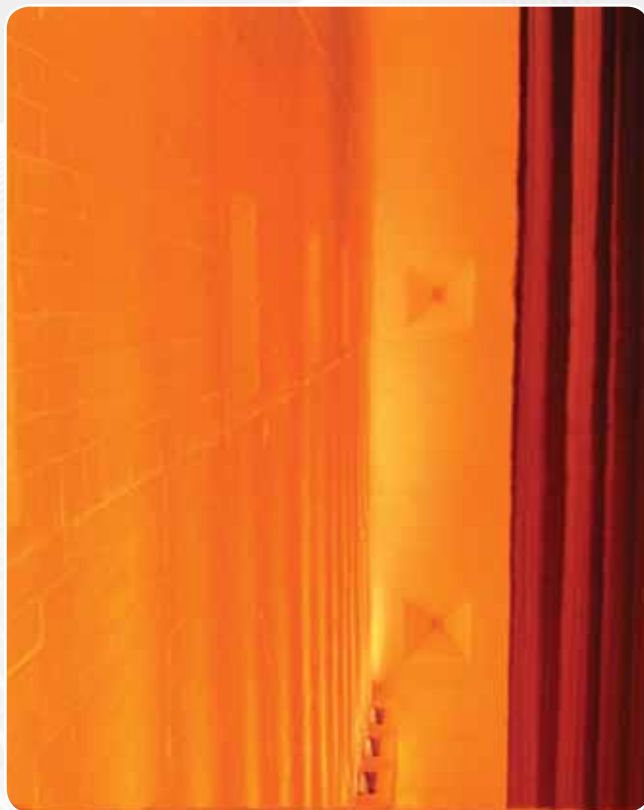
GLSF Enhanced Jet Burner, Horizontally Mounted
