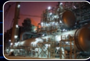
World's largest SRU tail gas incinerator with firetube waste heat boiler and steam drum. One of nine similar systems supplied by Zeeco.
