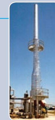
Vertical tail gas incinerator.
