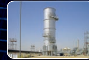
Vertical SRU tail gas incinerator.
