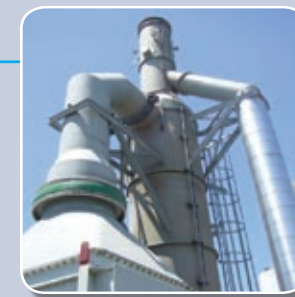
Vertical tail gas incinerator with hot oil heater for waste heat recovery purposes.
